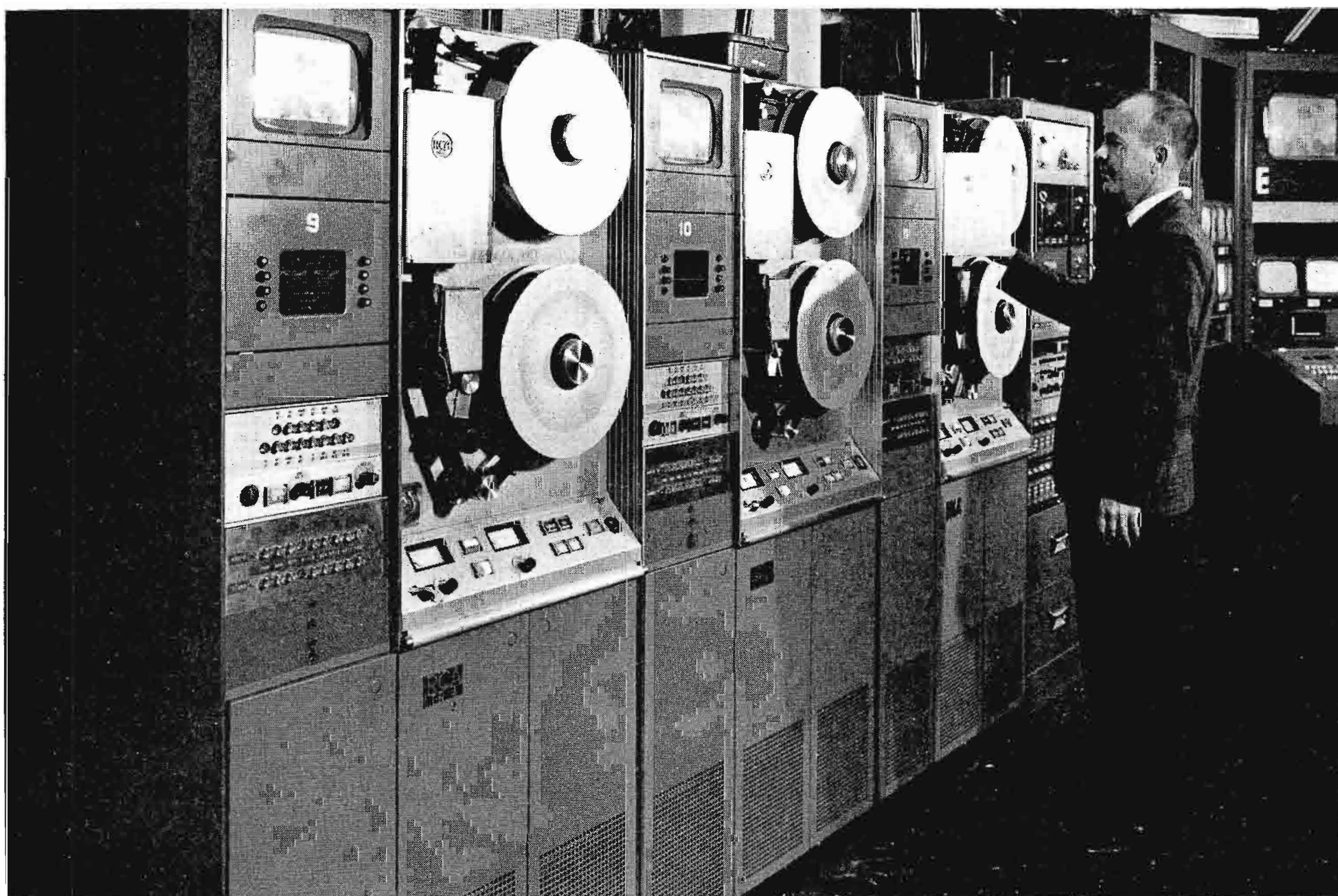
FIG. 2. Typical installation at WMAL-TV keeps group of TR-4 recorders busy on color programs and color commercials.
